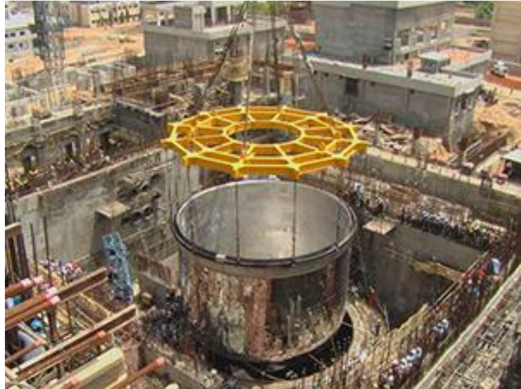
Prototype Fast Breeder Reactor (PFBR) at Kalpakkam, India
